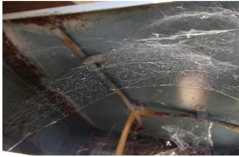
Figure 30. Tangle web/ Cobweb
